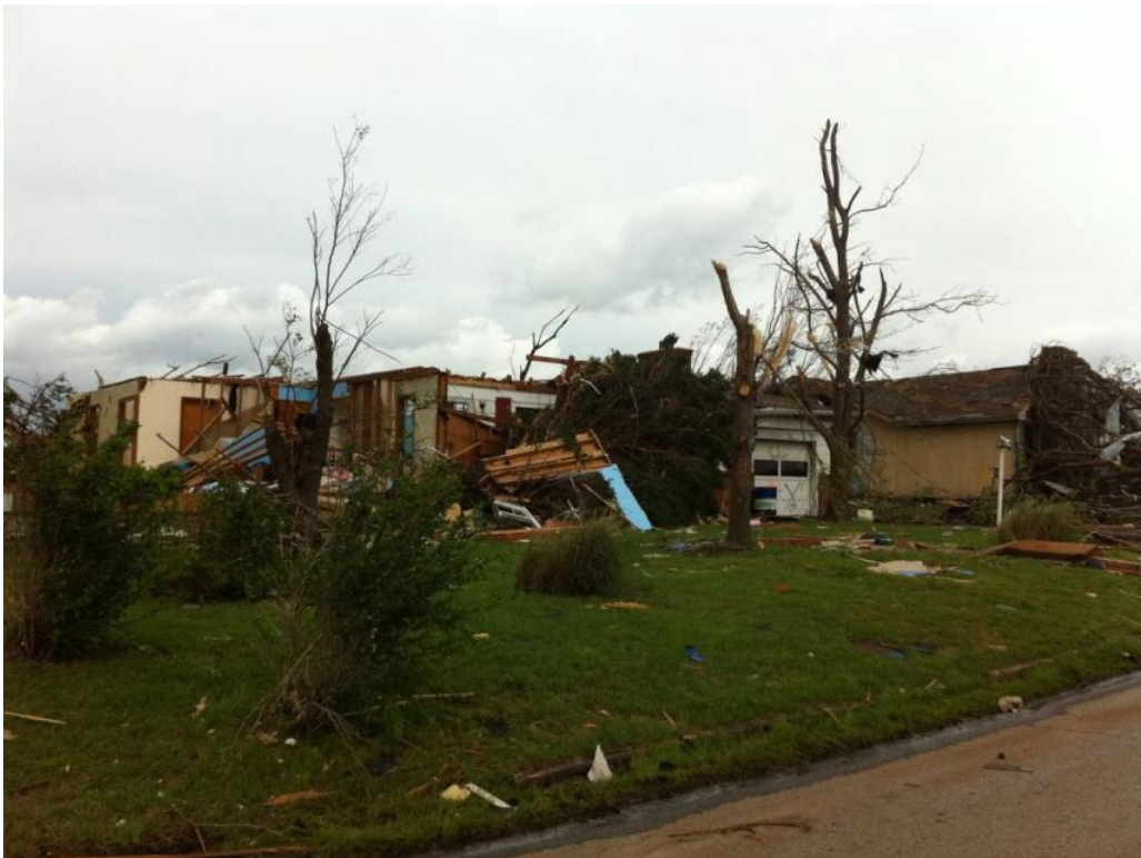
Figure 8.3 Roof and wall partially damage at the outer edge of the Joplin tornado path
